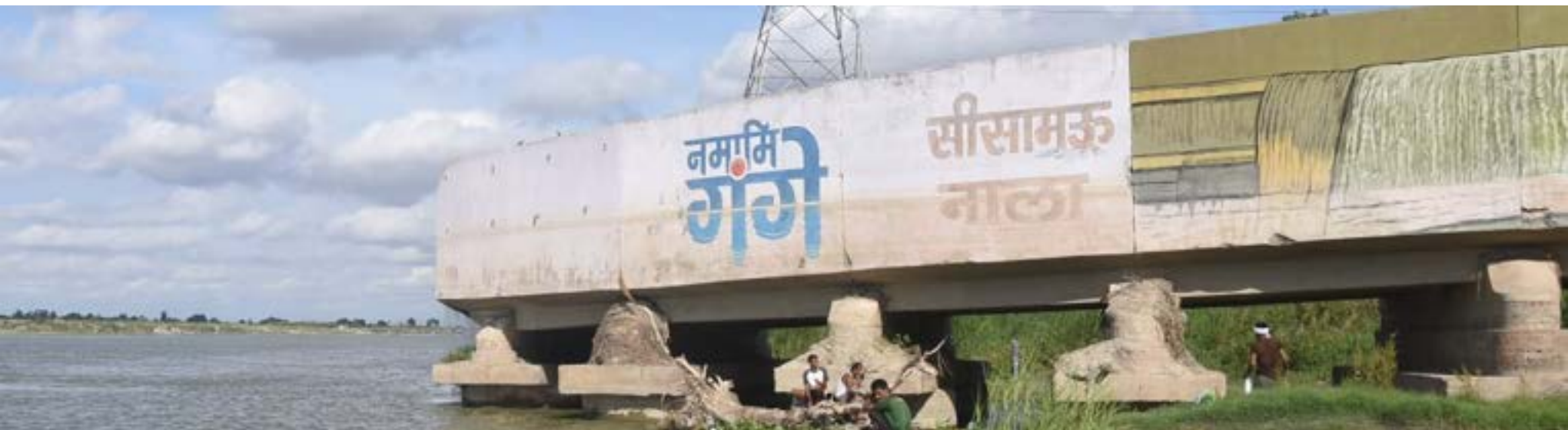
The infamous 140 MLD Sisamu Nala before and after the tapping (Source - NMCG)
